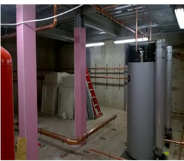
Boiler installation to Plant room to serving Block B, C and E
